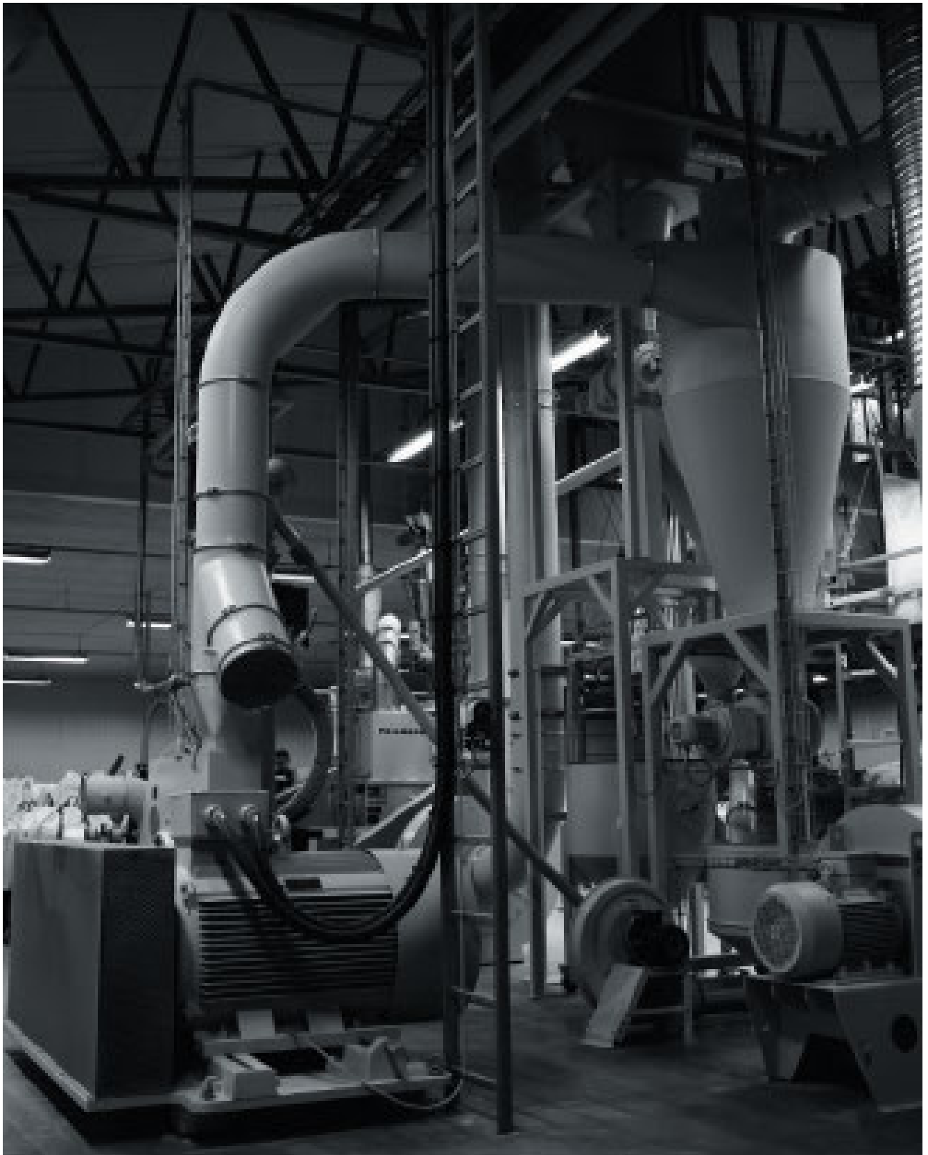
Bolon On-Site Recycling Plant
